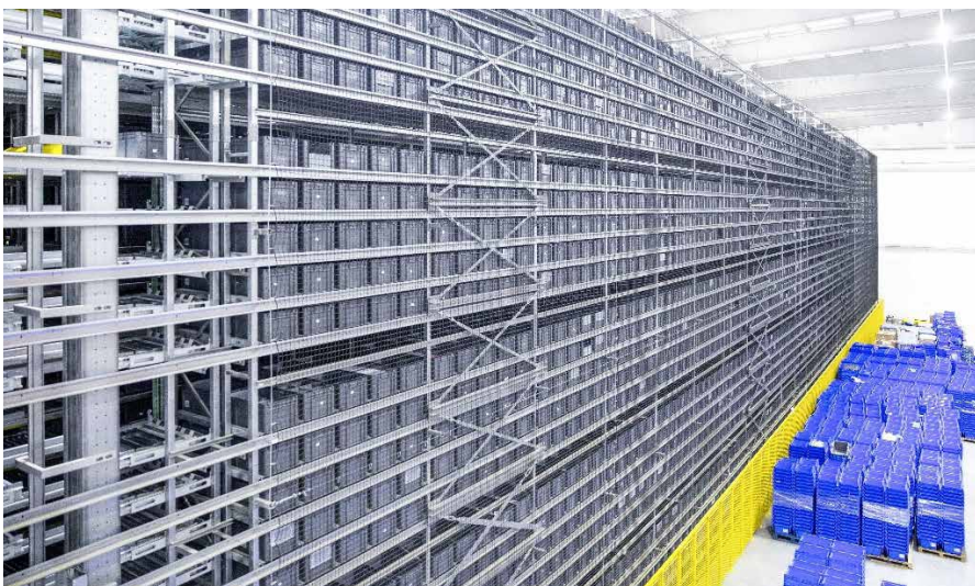
WAMAS® allows tracking for the entire material workflow using a single software suite.
